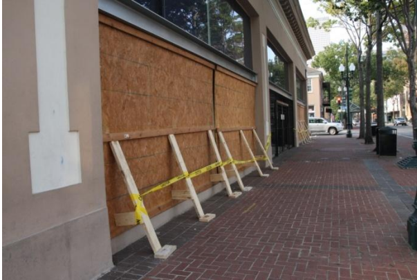
Figure 3. Boarded up glass store front in Louisiana (FEMA News Photo)
